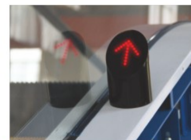
运行方向指示 Running direction indication
